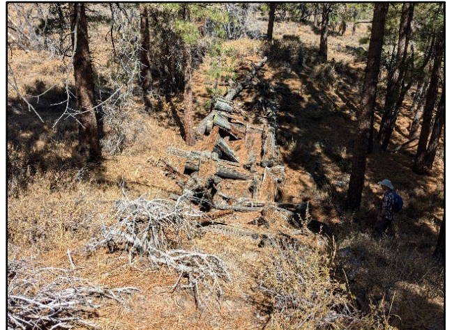
This collapsed “trestle” on the Verdi Lumber Company Railroad is really just a pile of logs that fill a ravine with tracks that once ran across the top of the pile.
